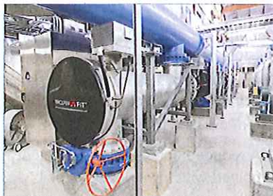
Figure 2. Four closed vessel reactors were installed post-membranes for this 894 L/s (20.4 MGD) water reclamation plant.
