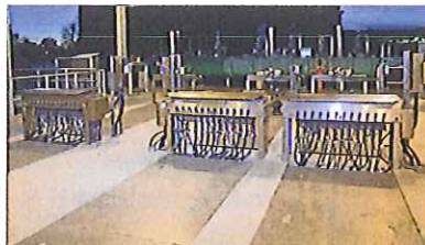
Figure 1. This 732 L/s (16.7 MGD) water reuse plant installed an open channel UV system.
