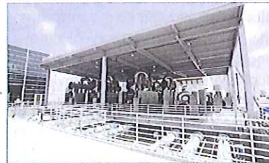
Figure 4: The Orange County Water District's 4381 L/s (100 MGD) Groundwater Replenishment System employs UV-oxidation as a final barrier for pathogens, nitrosamines, pharmaceuticals, industrial chemicals and other contaminants.
